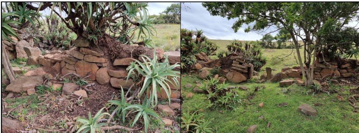
Figure 5-24: View of a dilapidated stone walls at Site EXIGO-NWEF-HP27.
