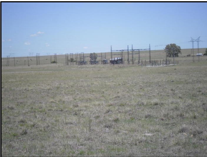
Figure 11. Substation that power will feed into.
