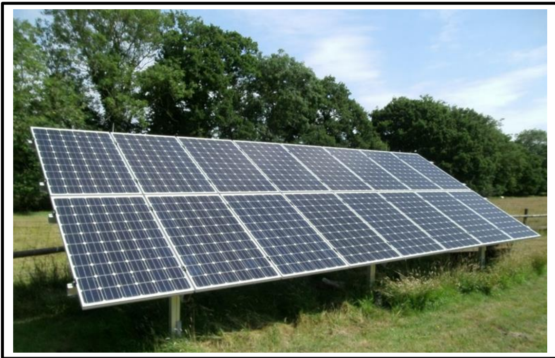
Figure 1.2: Ground mounted solar panel
