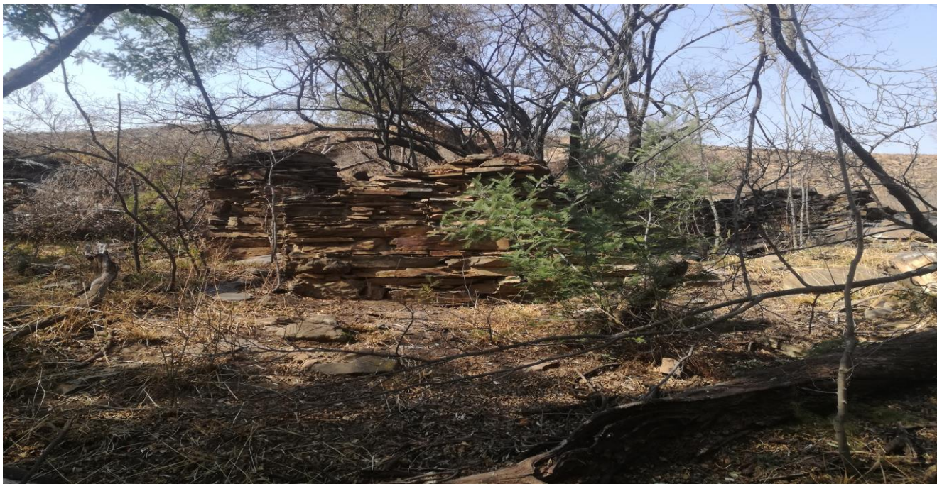
Plate 16: Photo 16: View of one structure closer to the river (Photograph © by Author 2018)
