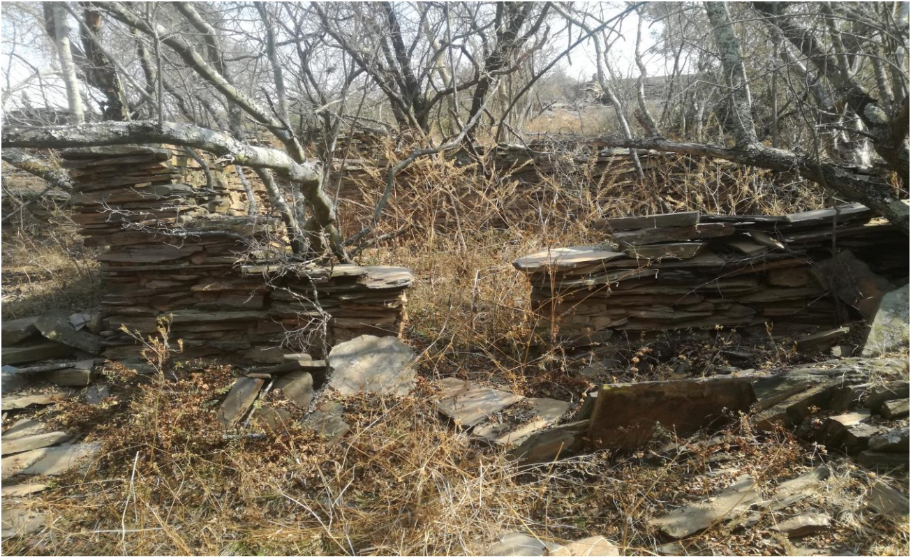
Plate 25: Photo 25: View of structure with trees which are likely to destroy the walls should they be an accidental fire (Photograph © by Author 2018)
