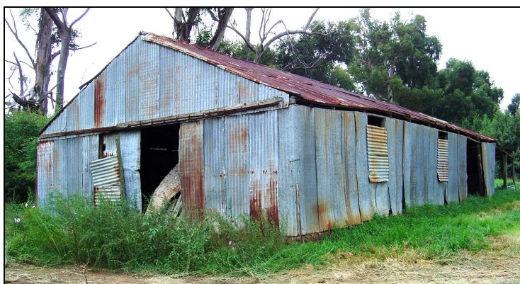
Fig.20 The old in a bad state of deteriorated.
