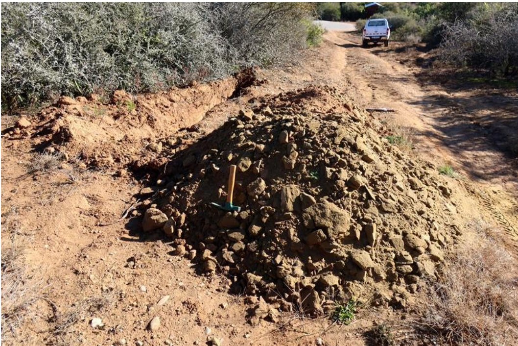
Figure 11: Test trench along the track defining the north-eastern edge of the project area. The excavated material is mainly friable, greenish-brown, weathered sandstone of the Kirkwood Formation (Hammer = 26.5 cm).
