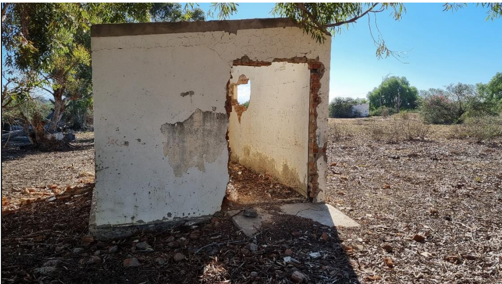
Figure 23. View of the of the remains of the school buildings.
