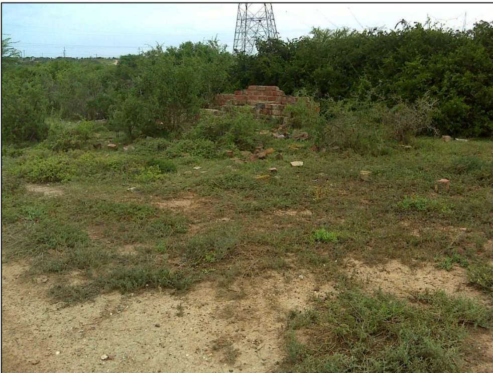
Figure 15. View of the degraded built environment structure situated adjacent to the proposed pipeline route (BE1).
