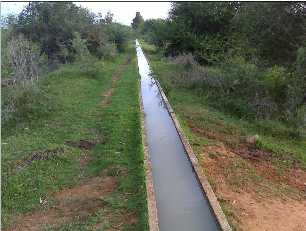
Figure 18. View of a narrow cement canal located along the route for the proposed pipeline.
