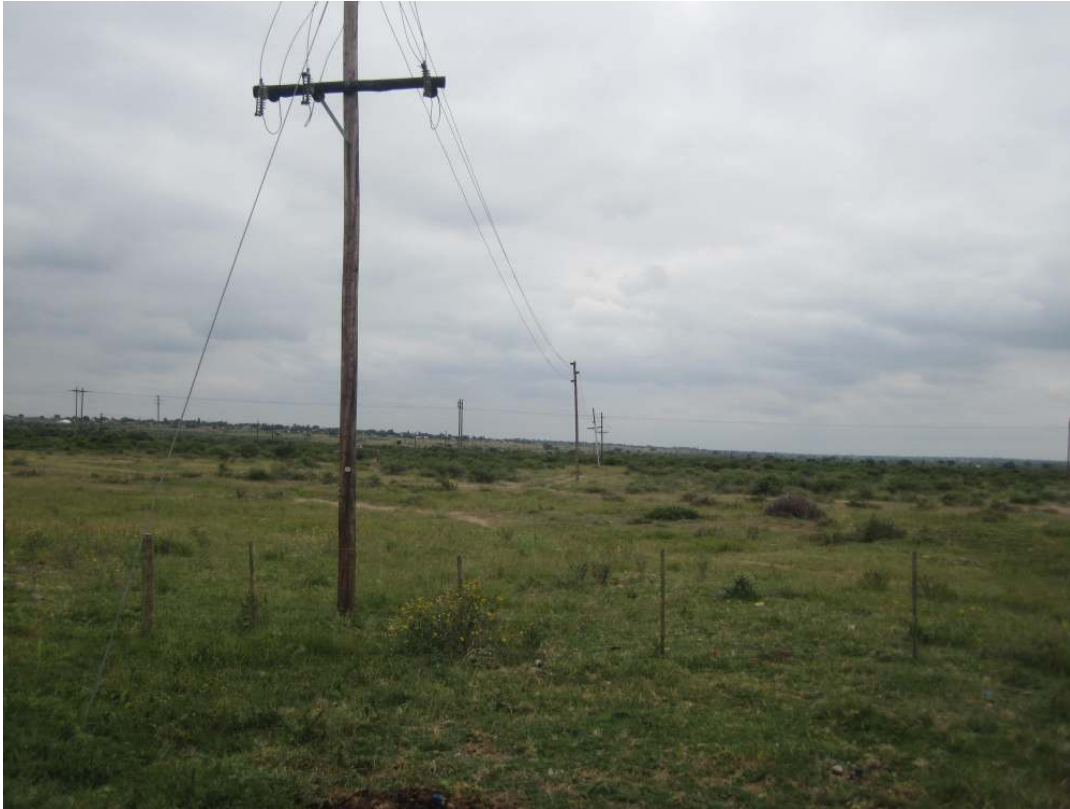
Photo 3: View of the power lines across the site.
