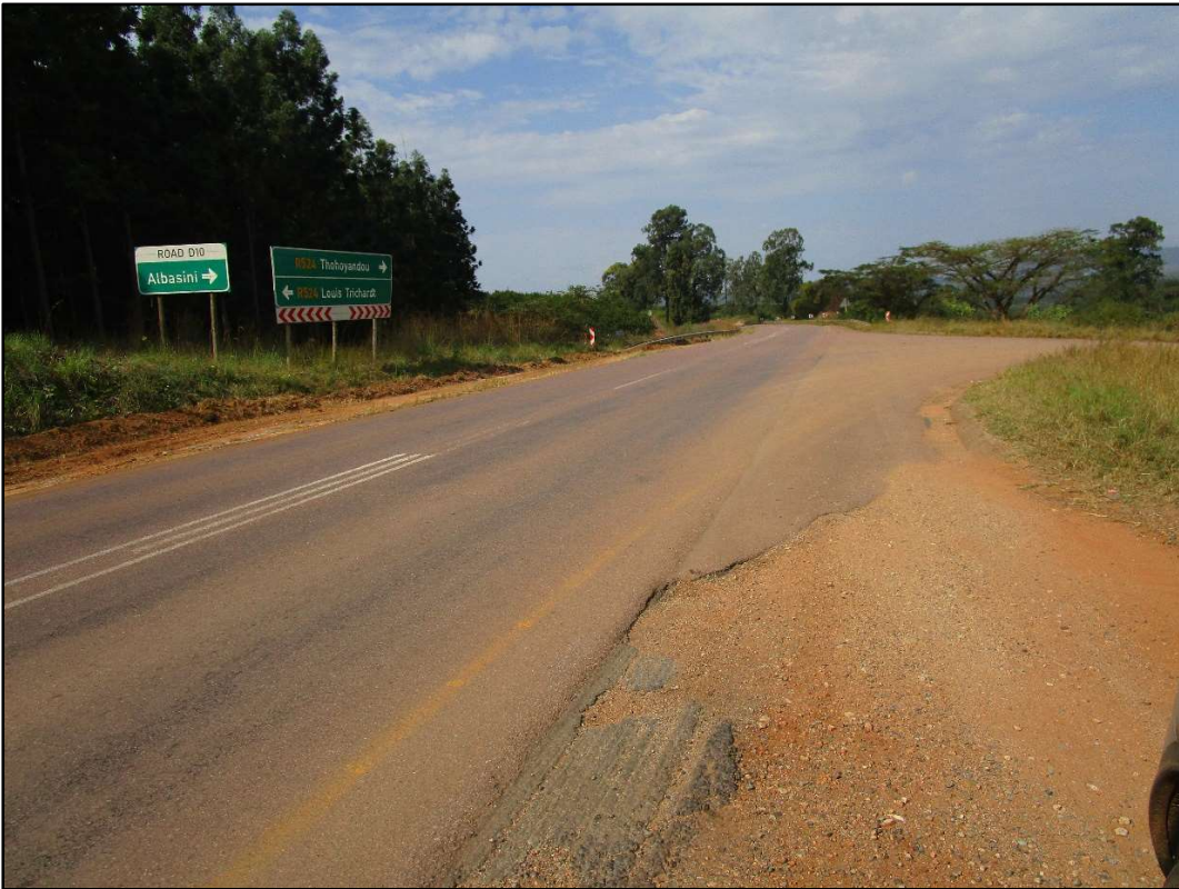
Figure 6. A view of the start of the upgrade of R524 – easterly direction. It shows the turnoff to Albasini dam. Position 1 on figure 4.
