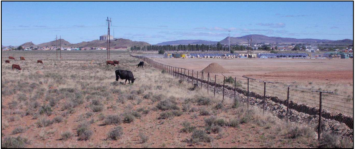
Figure 29: View westwards towards the town of De Aar showing a solar energy facility under construction between the site (left of the fence) and the R48 (out of picture to the right).
