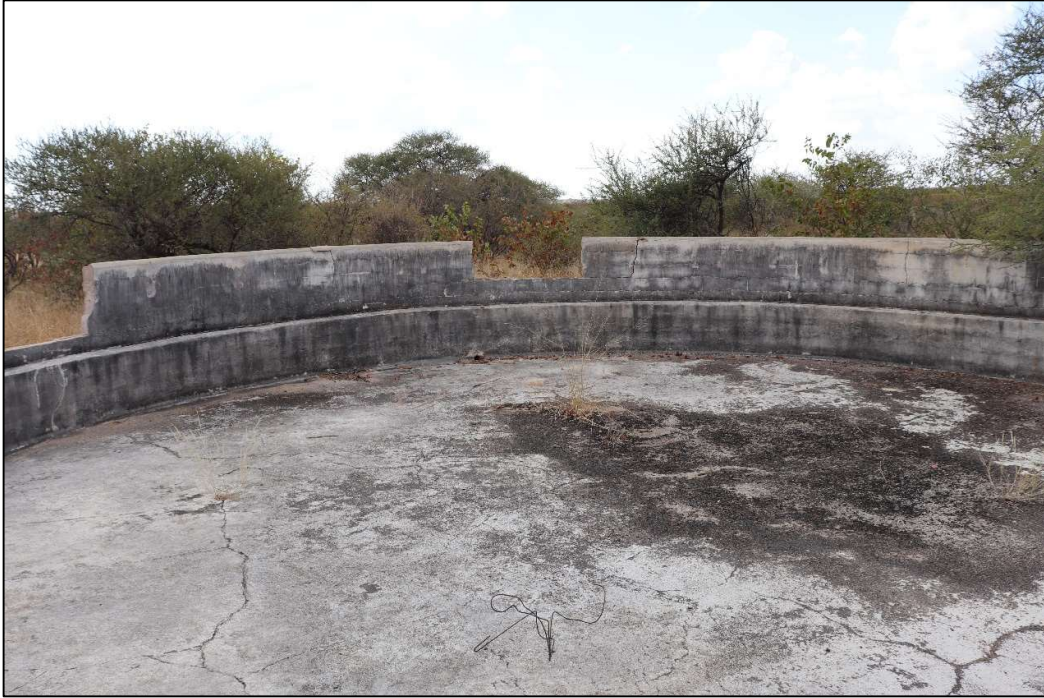
Figure 12: A concrete reservoir on the southern section of the Kalope River bank
