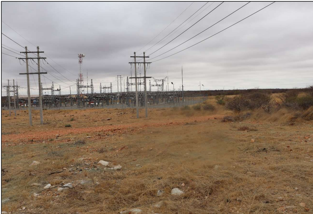
Figure 14: View of the Substations
