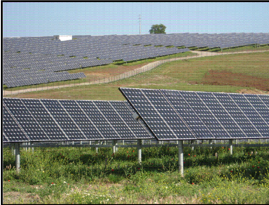
Figure 1.2: Stationary solar PV panels.
