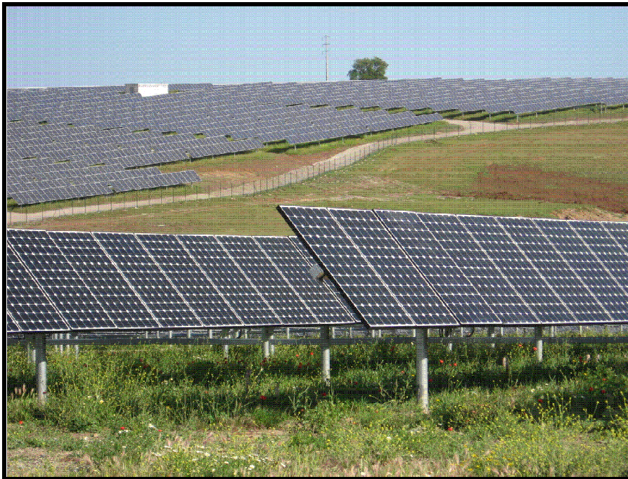
Figure 1.2: Stationary solar PV panels.
