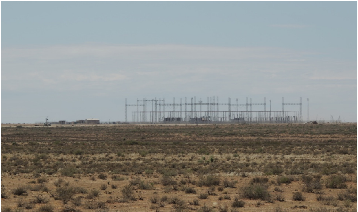
Figure 12: Photograph 1 looking south from the proposed power line route towards the Eskom Nieuwehoop substation.
