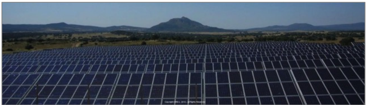
Figure 3: Photographic example of a typical PV energy facility ( www.hawaiiirenewableenergy.org/Villamesias2 )
