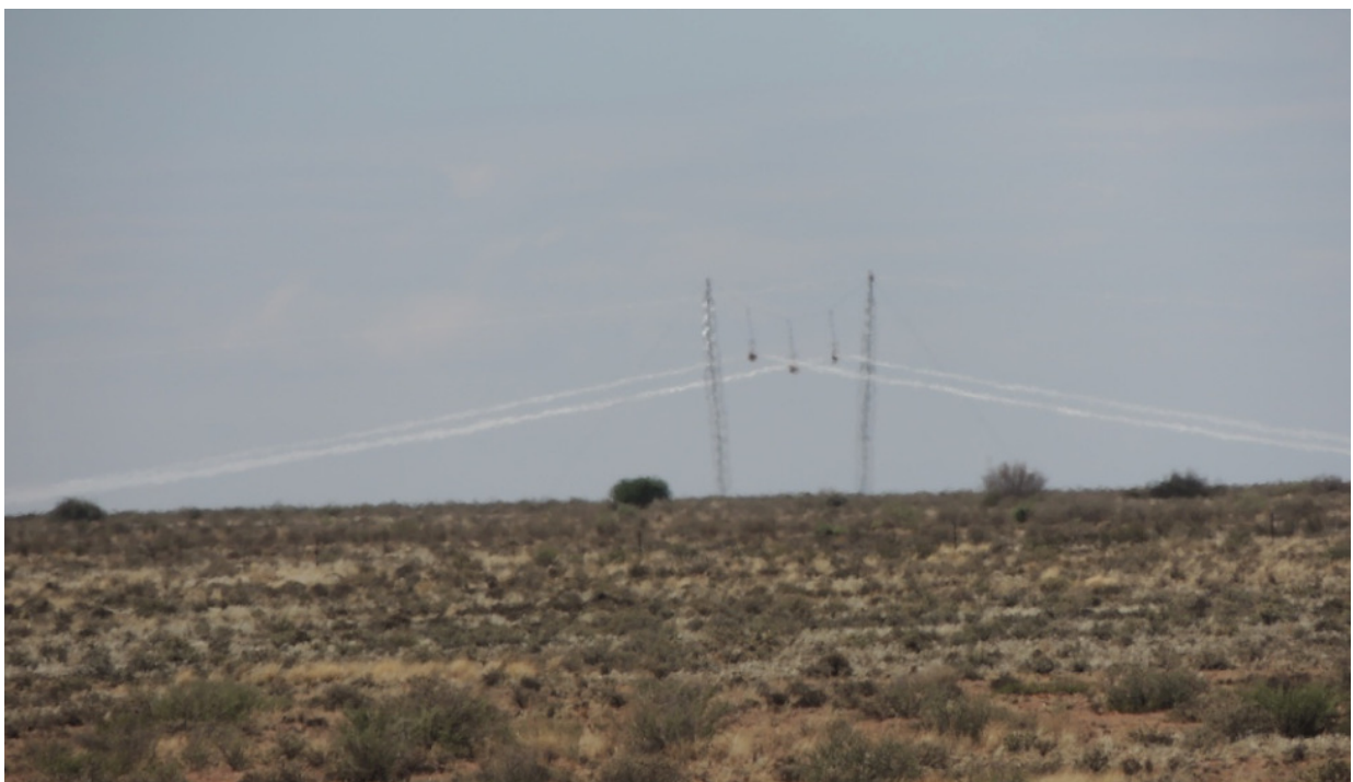
Figure 13: Photograph 2 looking south of Eskom power line corridor that links to the Nieuwehoop substation.
