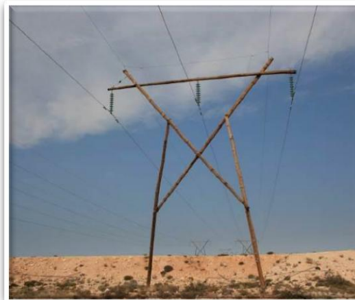
Example of an existing 132 kV transmission line (Source: VRMA)
