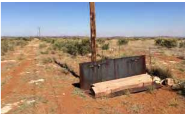
Figure 16: Example of Eskom power pole base support on the proposed site.
