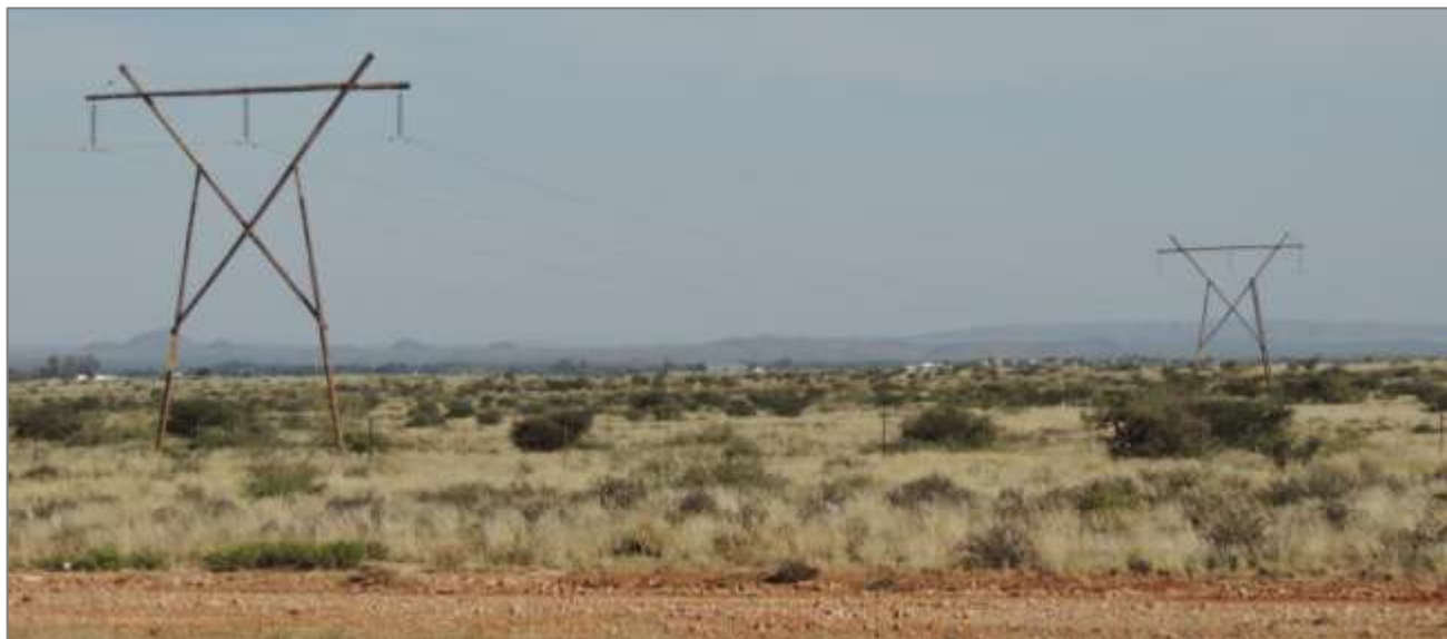
Figure 9: Photograph of the existing transmission lines located to the south of the proposed site.
