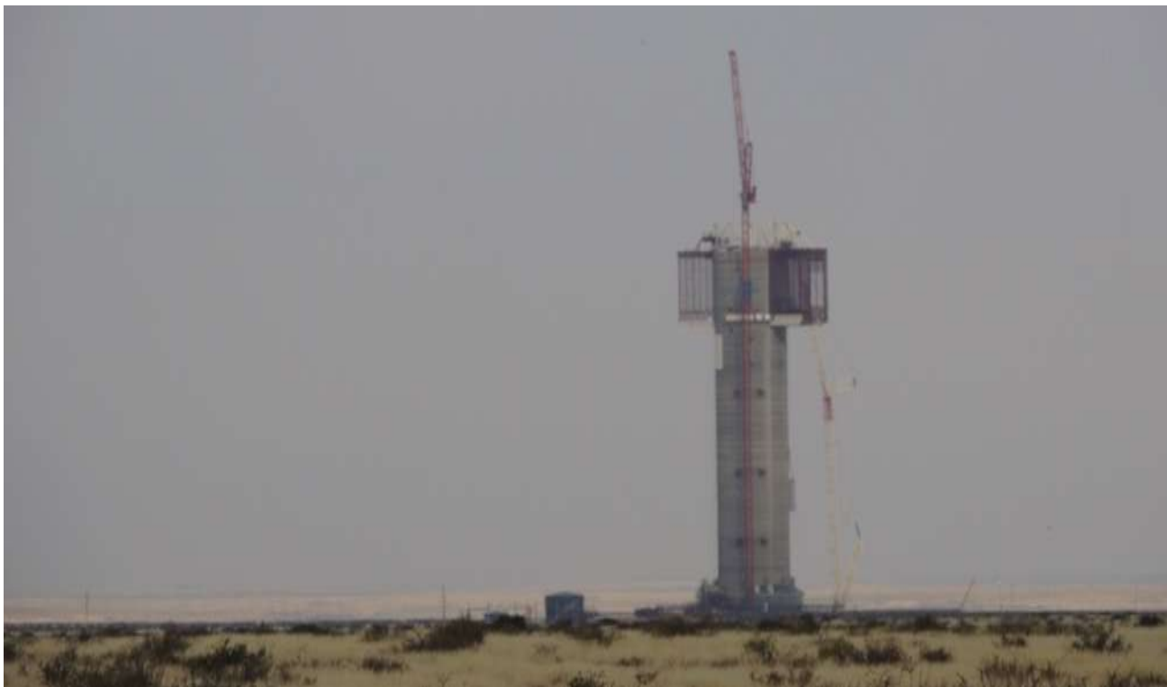
Figure 7: View of Khi Solar One CSP under construction as seen from the N14.
