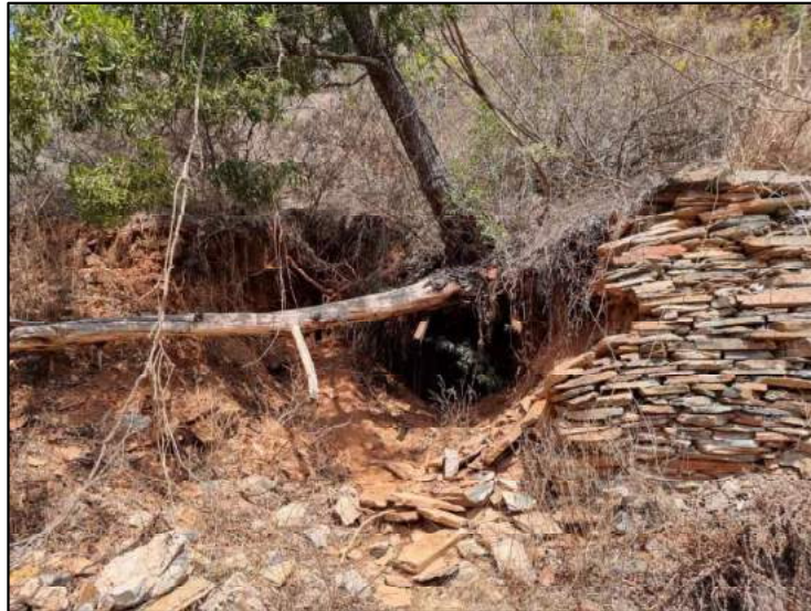
Figure 6-45: View of a partially collapsed adit in the CDM Mining Area at the extant Morgenzon Mine.
