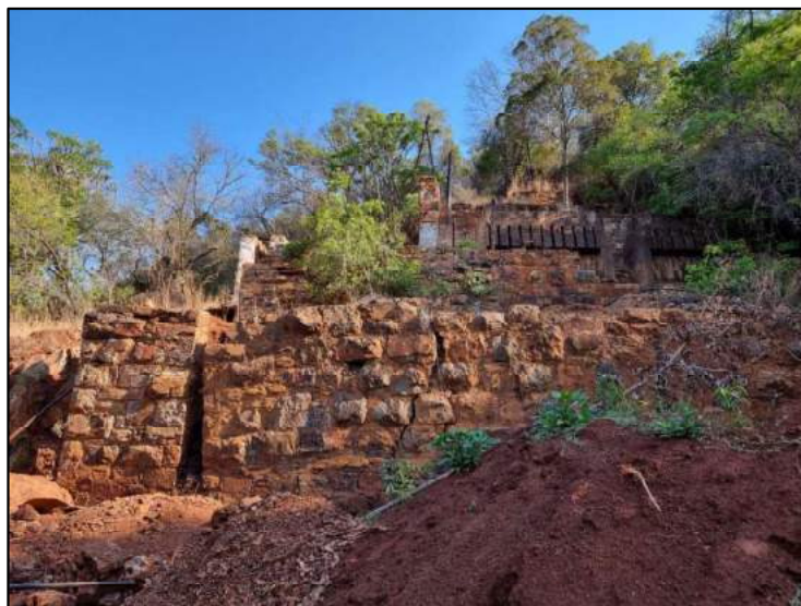
Figure 6-29: View of the dilapidated remains of a MET plant in the Frankfort Mining Area at NH-TGME-2430DC-10.
