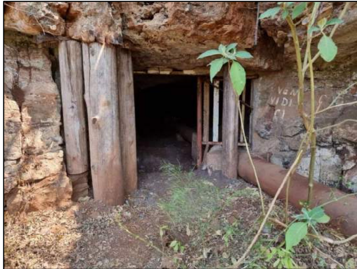
Figure 6-10: View of a Historical / extant drainage shaft in the Beta North Mining Area
