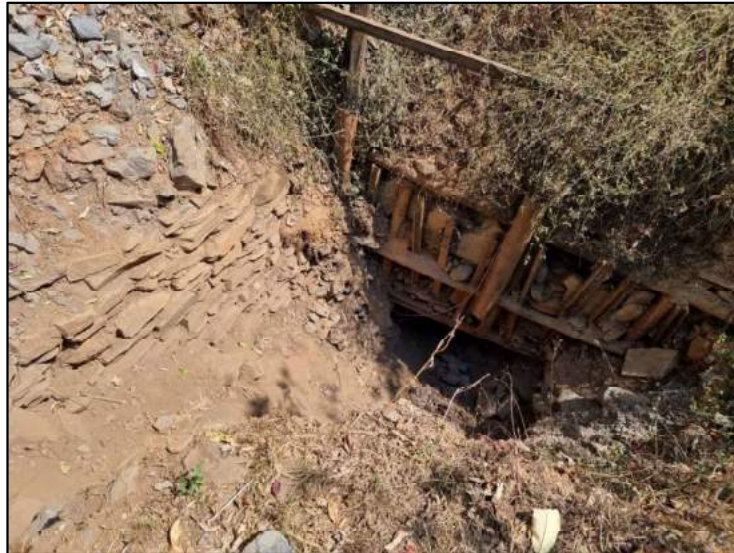
Figure 6-41: View of a collapsed Historical Adit in the CDM Mining Area at the Upper Dukes mine.
