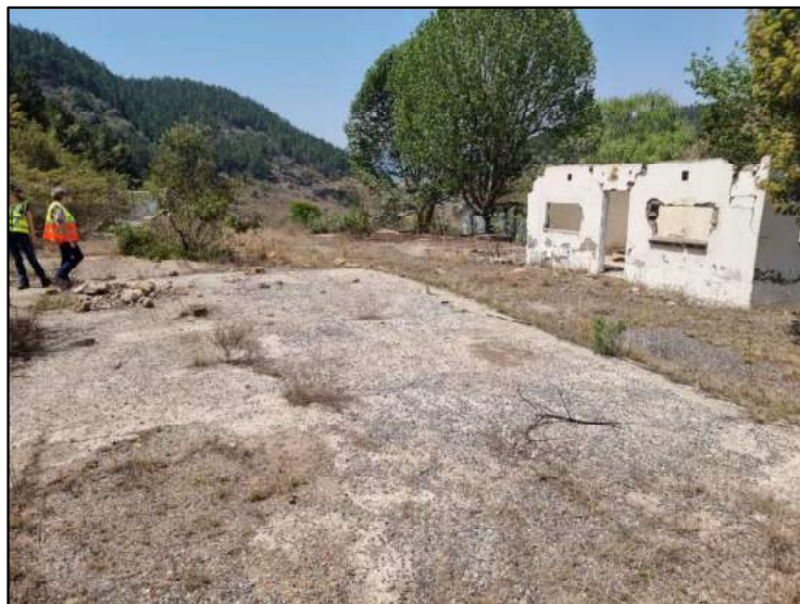
Figure 6-35: The former TGME offices in the CDM Mining Area at the Morgenzon mine.
