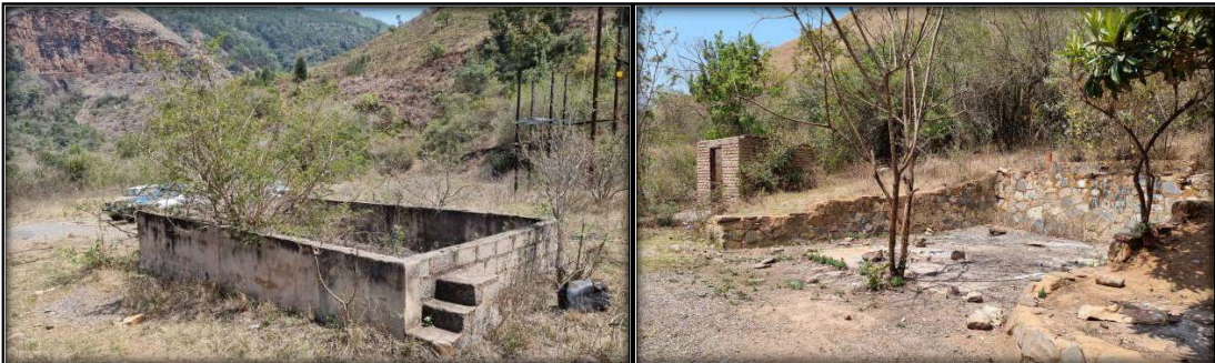
Figure 23: Neglected site of the Morgenson site infrastructure.
