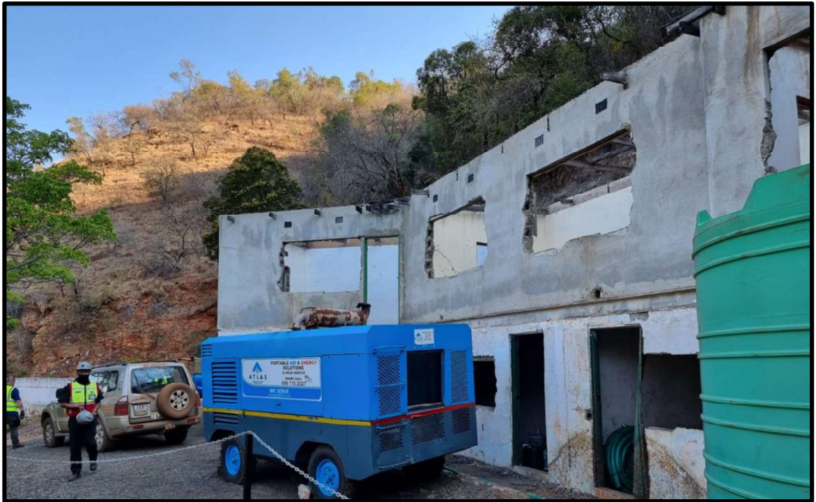
Figure 18: Neglected Frankfort mine Offices
