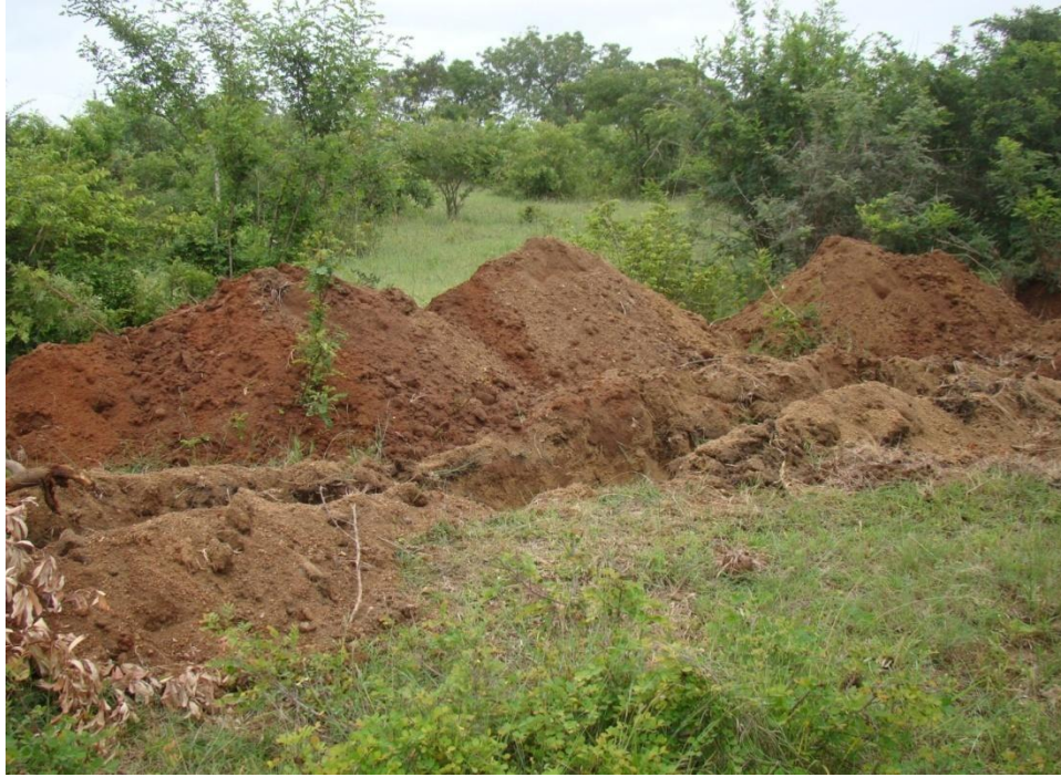
Fig. 9: An excavated section on the entire northern section for a water pipe to a cultural village.
