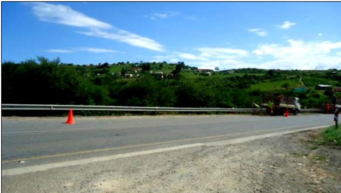
Fig 24 R61 over Mngazi River bridge showing access road to be re-aligned on east bank in foreground
