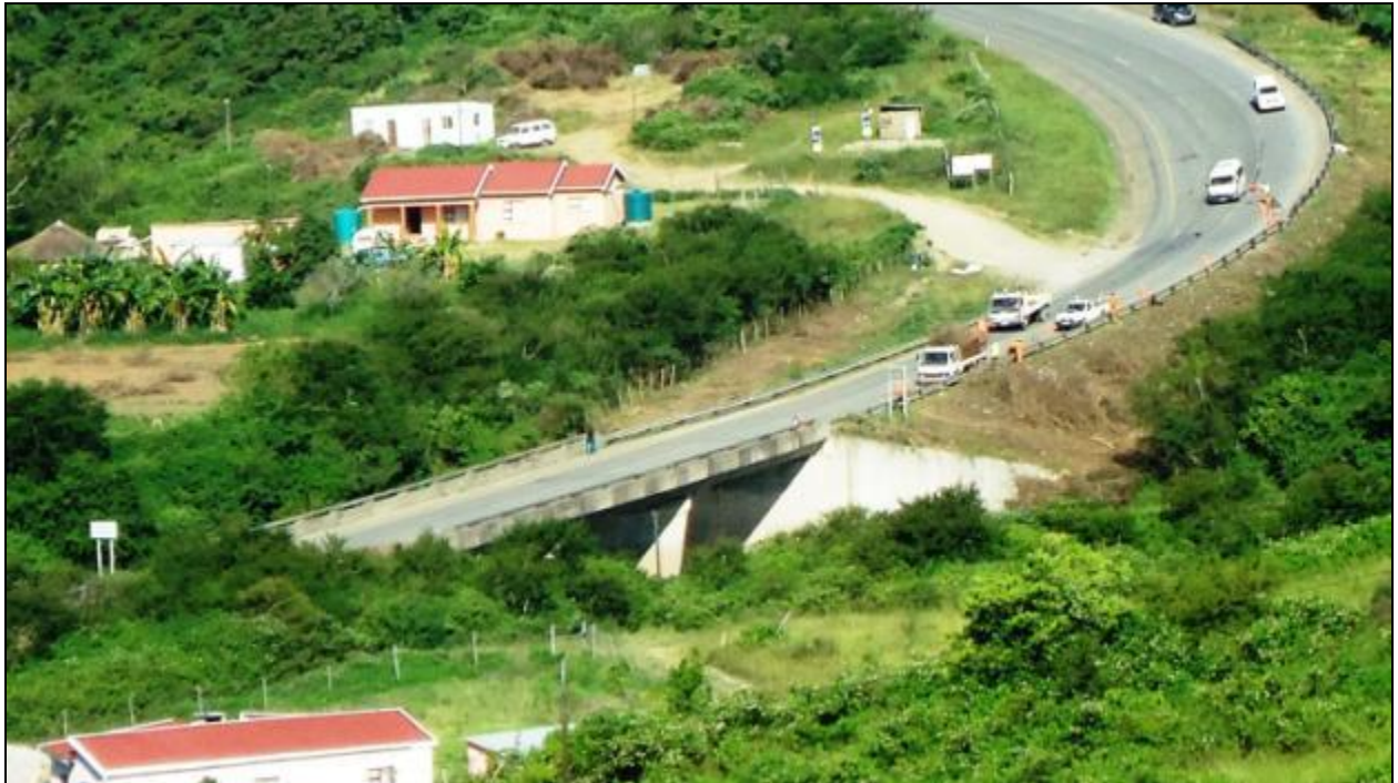
Fig 1 View of Mngazi River bridge from west bank looking towards the east bank March 2014.
