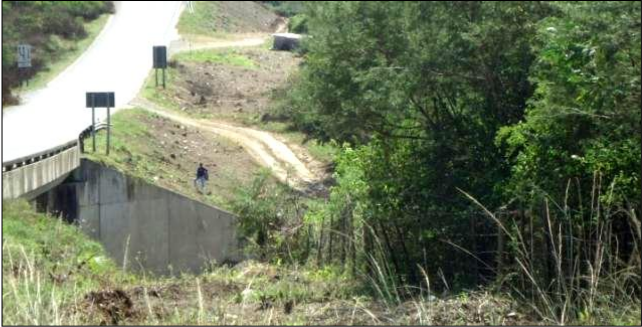
Fig 13 Bush cleared on east bank of Mngazi River bridge looking north-west S31° 36'34.73"; E029° 24'18.66"
