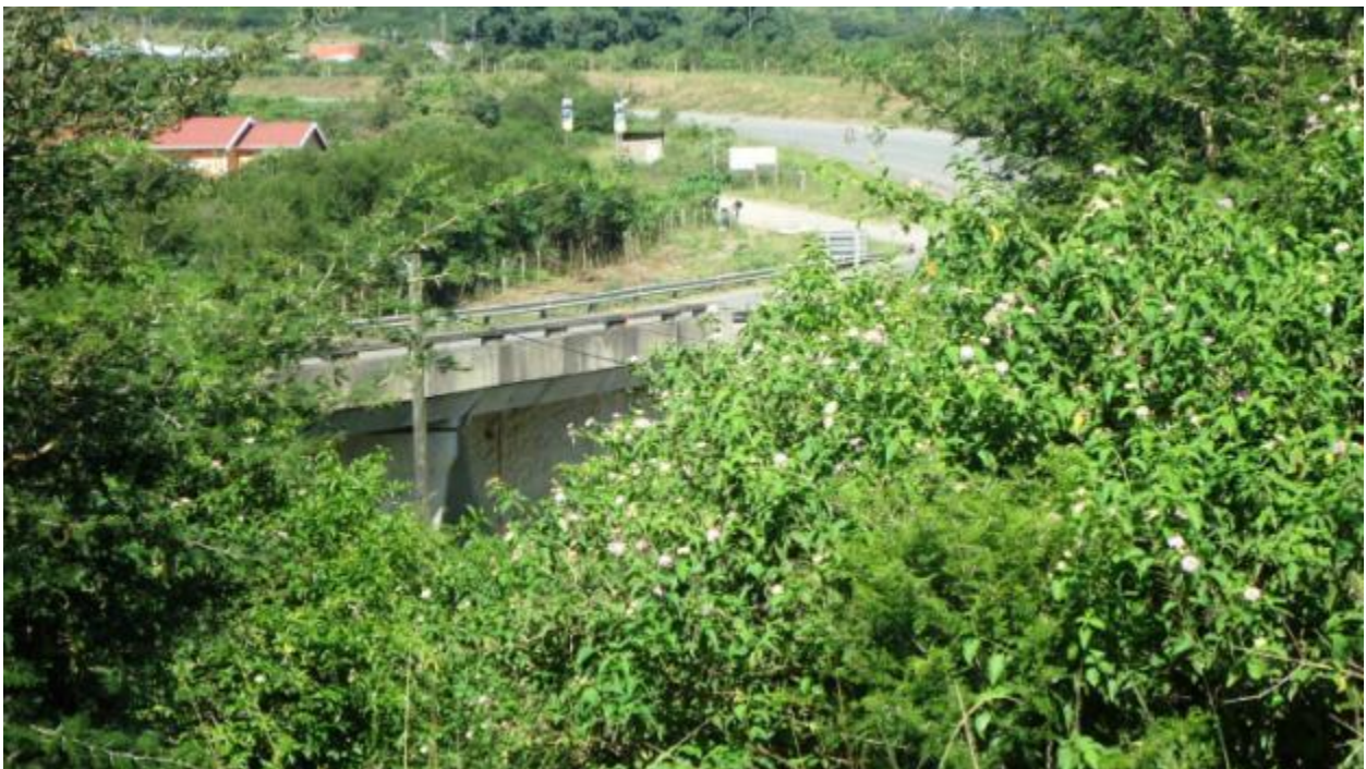
Fig 26 Mngazi River bridge almost obscured by lantana –west bank
