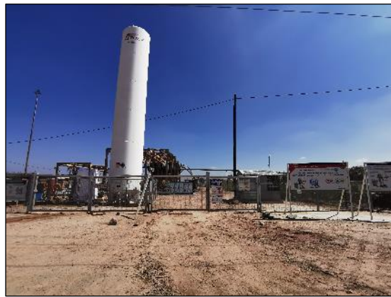
Figure 12 - View of the Brand A Pump Station
