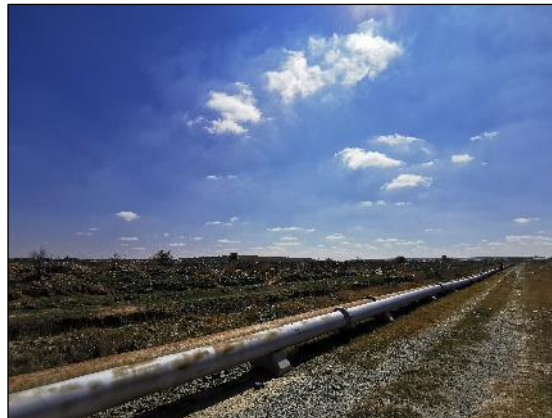
Figure 10 – Alignment along the service road with the large refuse dump located to the north
