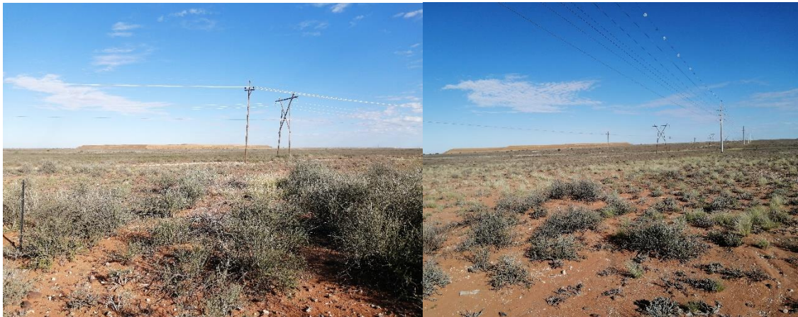
Figure 12 - Southern view of power line and site dam in the background on the farm Klipgats Pan 117
