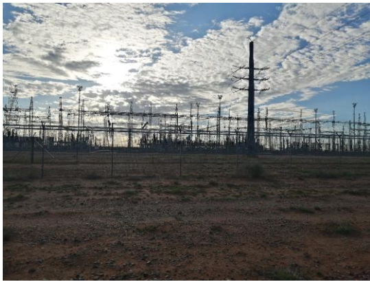
Figure 11 - Eastern view of Substation
