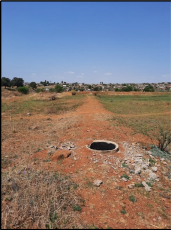
Figure 8.1. Existing degraded pipelines running towards the ground dams situated on the southern edge of the project area.
