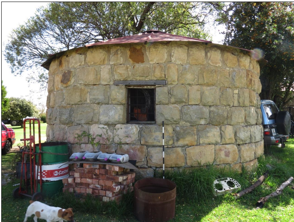
Figure 27 – Another view of the rondavel structure. Note the small rectangular window with wooden frame and lintel.
