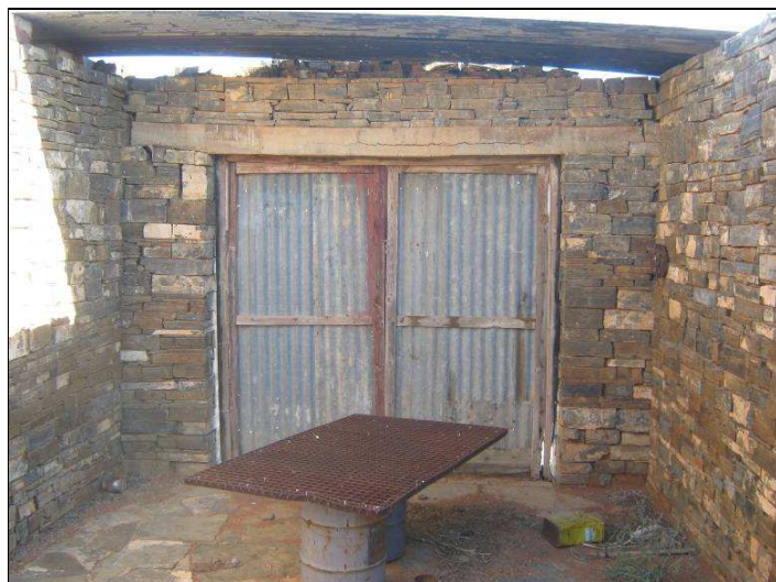
Figure 55: The inside of the large door to the cow shed. Note the concrete lintel.
