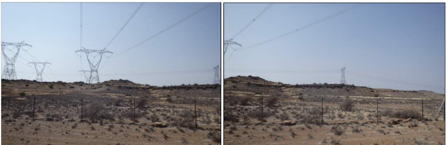
Figure 4.2: Existing grid infrastructure at the southern extent of the proposed grid connections
