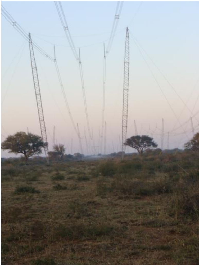
Figure 6: ESKOM powerline in the area. Note the servitude which has almost entirely been disturbed.
