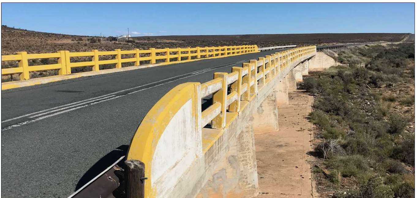
Figure 6.6 BTC07 - Bridge over the Soutpoot River (1958), northern side with basic structure evident
