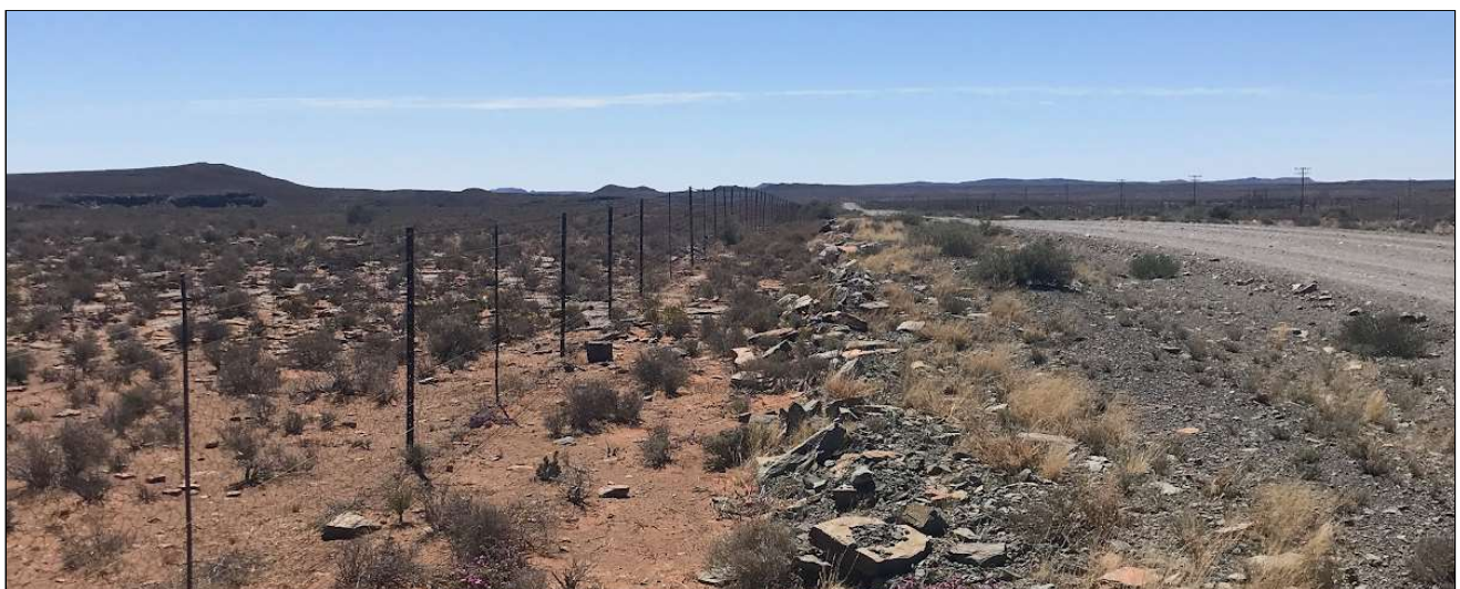
Figure 4.12: Contextual Images indicating the disturbed road surface
