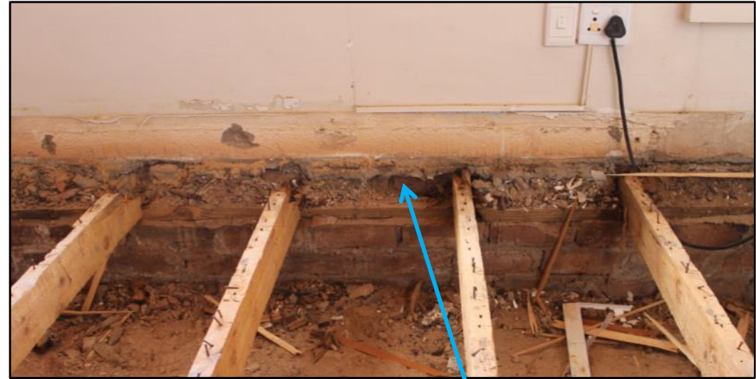
Figure 38: The floor beams are resting on a newly constructed wall in front of the original wall of the cottage. The enlargement shows red mud brick and red mud mortar.
