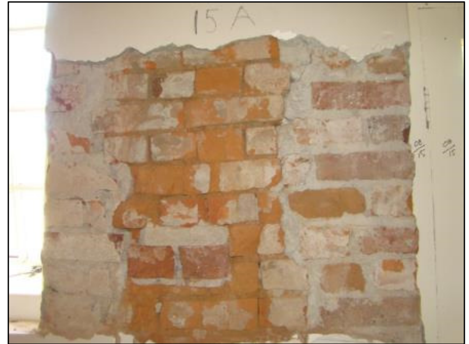
Figure 54: Section of walling between existing door and window shows the original wall of red brick and mud mortar and recent alterations to insert the window and door.
