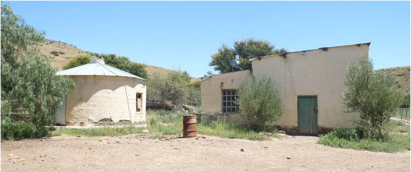
Early stone structure with later lean-to at the T-intersection, as shown on 1829 survey.
