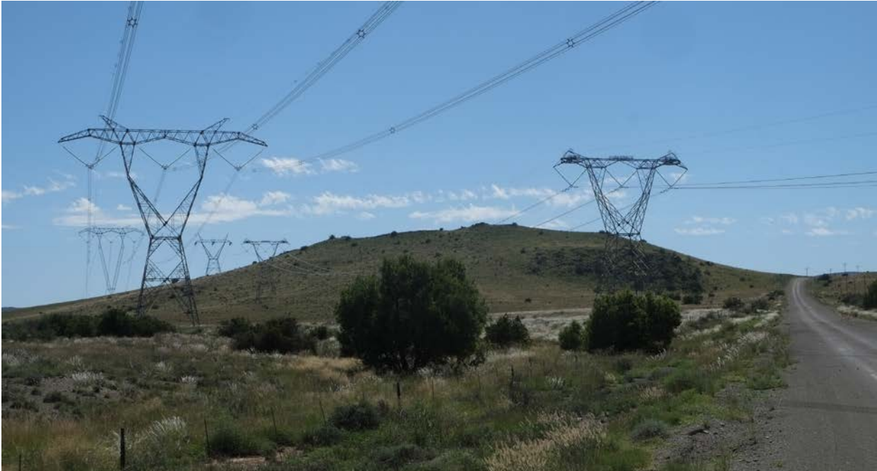
Powerlines cross at boundary of farm Belvedere.
