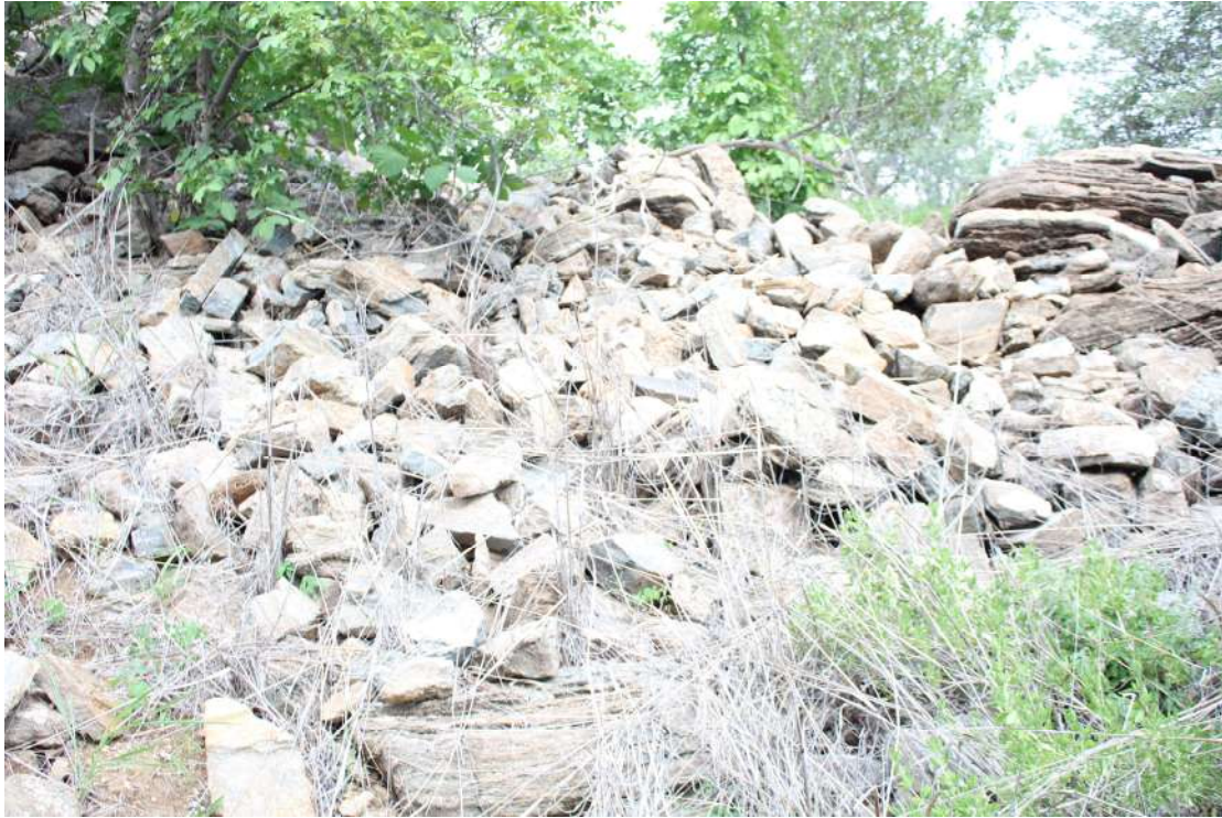
Figure 10: Collapsed stone wall on a rocky ridge
