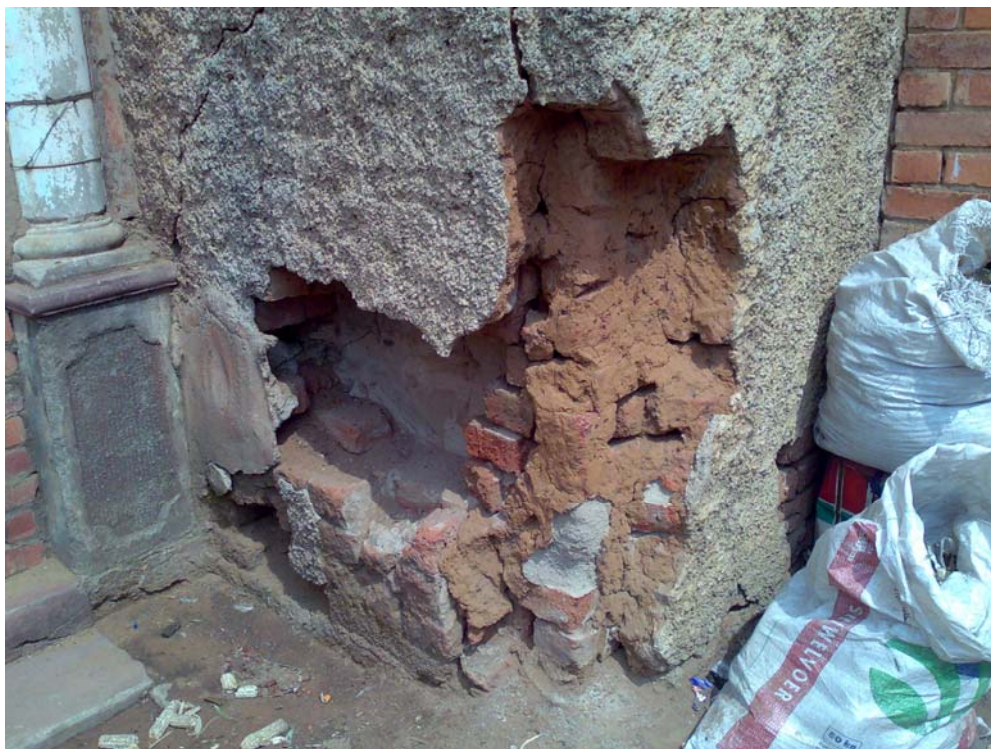
Figure 9: Unstable condition of some of the outer walling
