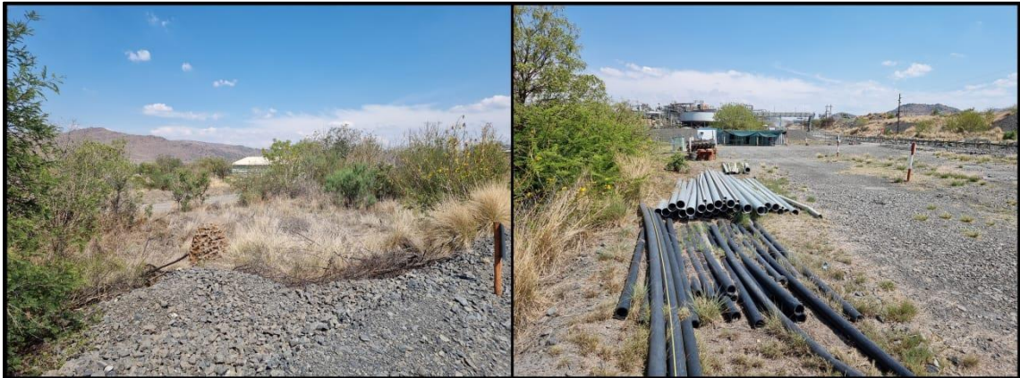
Figure 9: Views of the project area, note cleared surfaces and a temporary site office (right).
