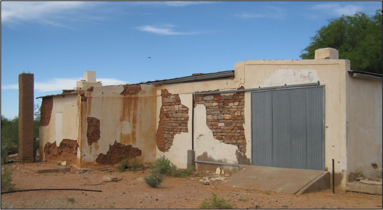
Figure 30: Dilapidated structure at the farmstead ay waypoint 526.
