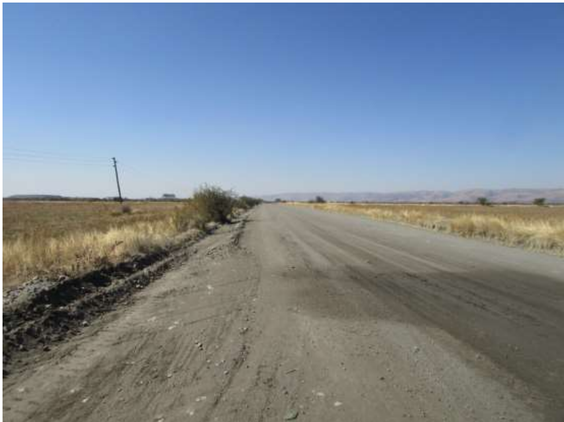
Figure 17: A view of the route or the new Pipeline. It will follow the existing Road reserve to a large extent and make use of existing connections.
