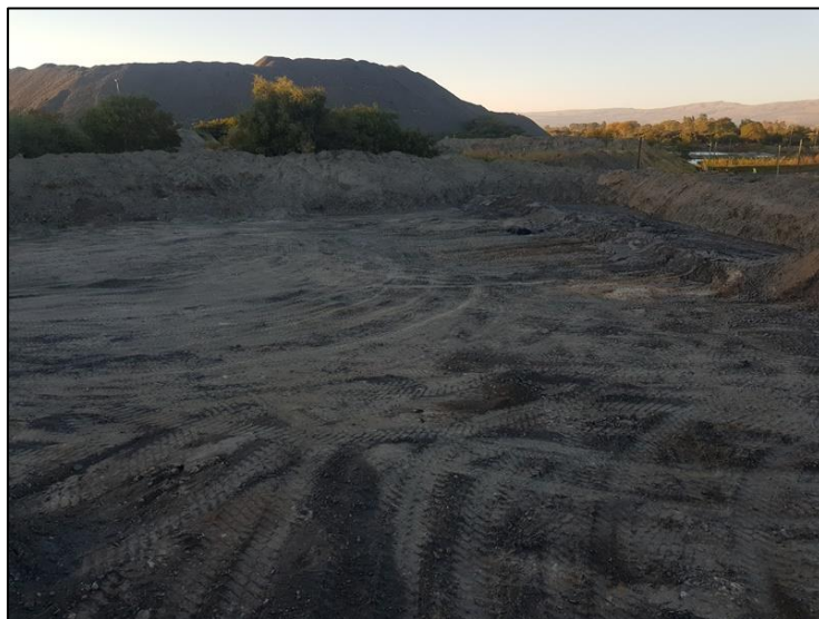
Figure 3-12: View of transformed surfaces at the site of the proposed waste rock dump extension.
