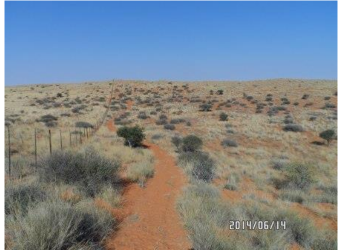
Photo 2: Typical view of pipeline route along farm road on Farm Cramond, with boundary fence to Farm Visch Gat to the left (Alternative route)
