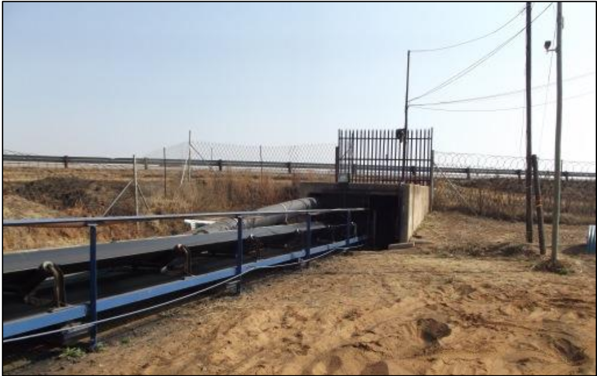
Fig. 3. Site KSO 2. Looking towards the north-west. The pipe will go underneath the N12 and proceed further south from here.
