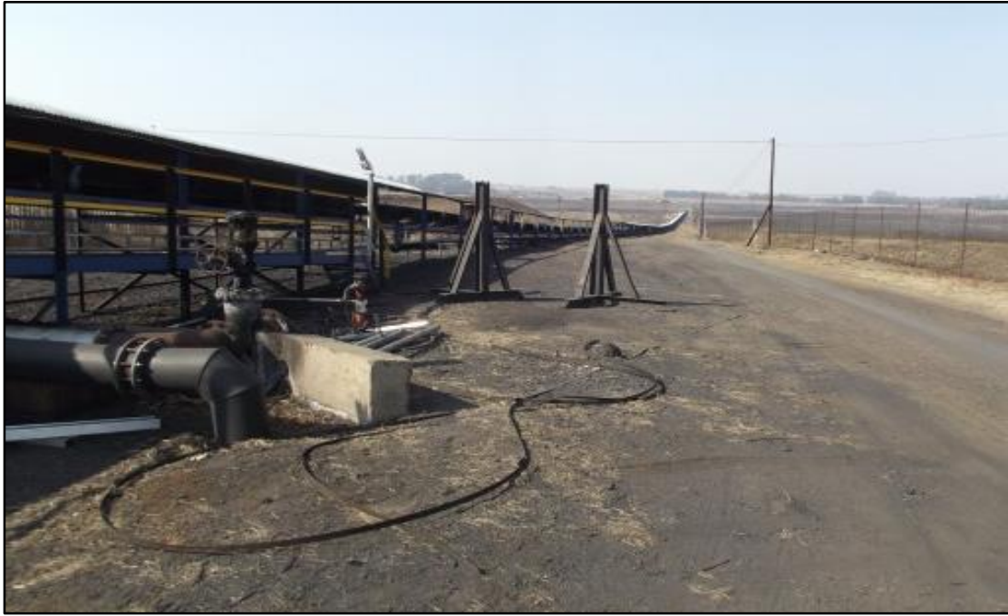
Fig. 1. Site KSO 1. Looking in a south-eastern direction, the pipeline will run parallel to the conveyor belt system.
