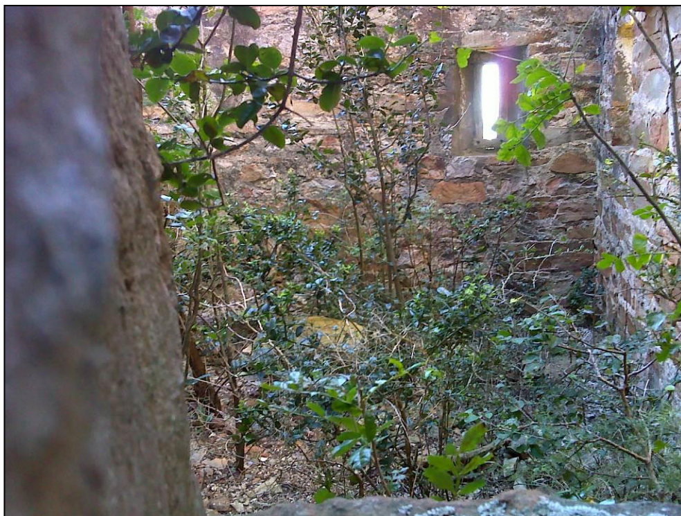
Figure 75. View of the overgrown vegetation cover inside the structure.
