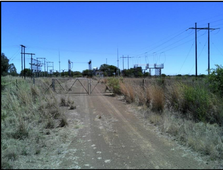
Figure 13: Heuningspruit substation that the project will feed into
