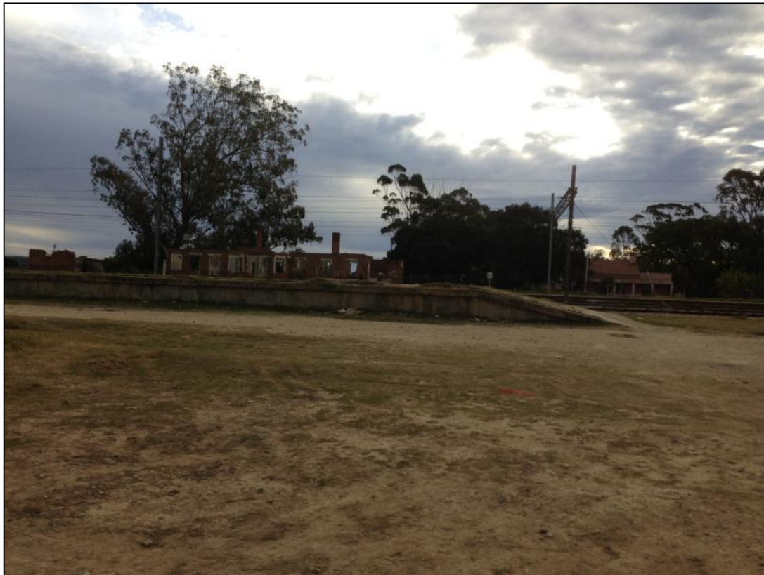
Figure 9. Dilapidated platform and station buildings
