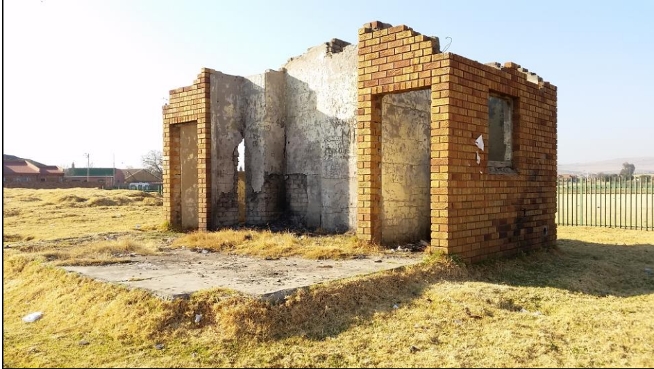
Figure 18: General view of ablutions, probably associated with the sport fields in the western section of the survey footprint
