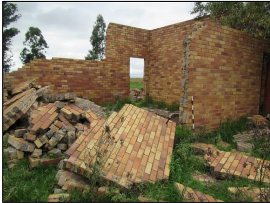
Figure 37 – c) Derelict brick structure at LES011
