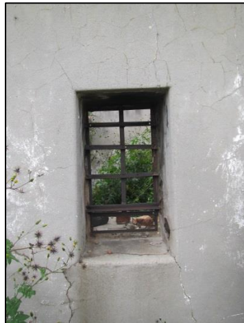
Figure 25 – Iron bars in window LES004
