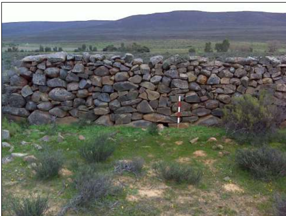
Figure 18. View of the dry packed stone wall (K-PLSW1) on the Farm Standvastigheid 210.
