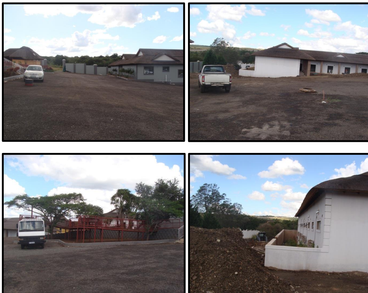
Figure 5 - 8: Construction was on-going on site, with large portions of the project in an advanced stage of completion. Top left (Fig.5) shows the entrance gate leading off of Thornetree Road. Various buildings were almost finished, leading off from a parking lot area (top right & bottom left, Fig.6 & 7). Looking east, showing the northern boundary wall with a large pile of shale in the foreground (Fig.8)
