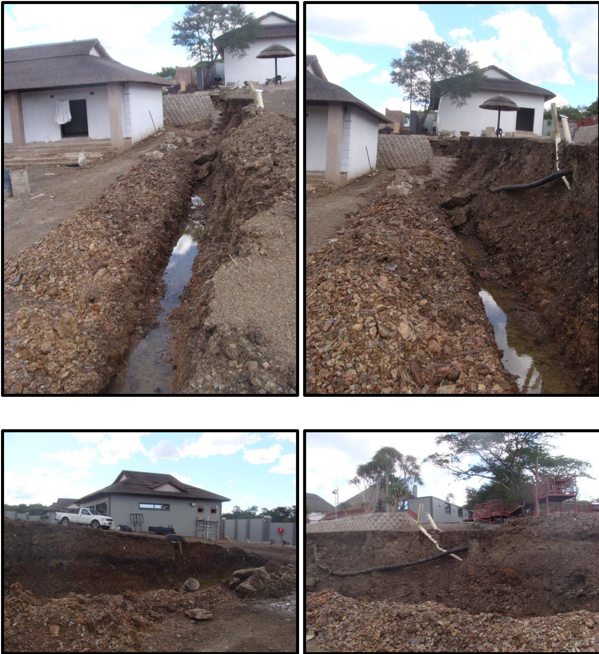
Figure 13 - 16: Whilst on site it was noted that an embankment was collapsing due to recent rainfall, which was being stabilised with cement blocks (top left & right, Fig. 13 & 14). This revealed that underground pipelines had already been installed and that the upper soil surface had been excavated to a depth of over 2 metres, indicating that the ground has previously been disturbed (bottom left & right, Fig. 15 & 16). A trench was dug below this embankment, which unearthed a considerable amount of Dwyka shale
