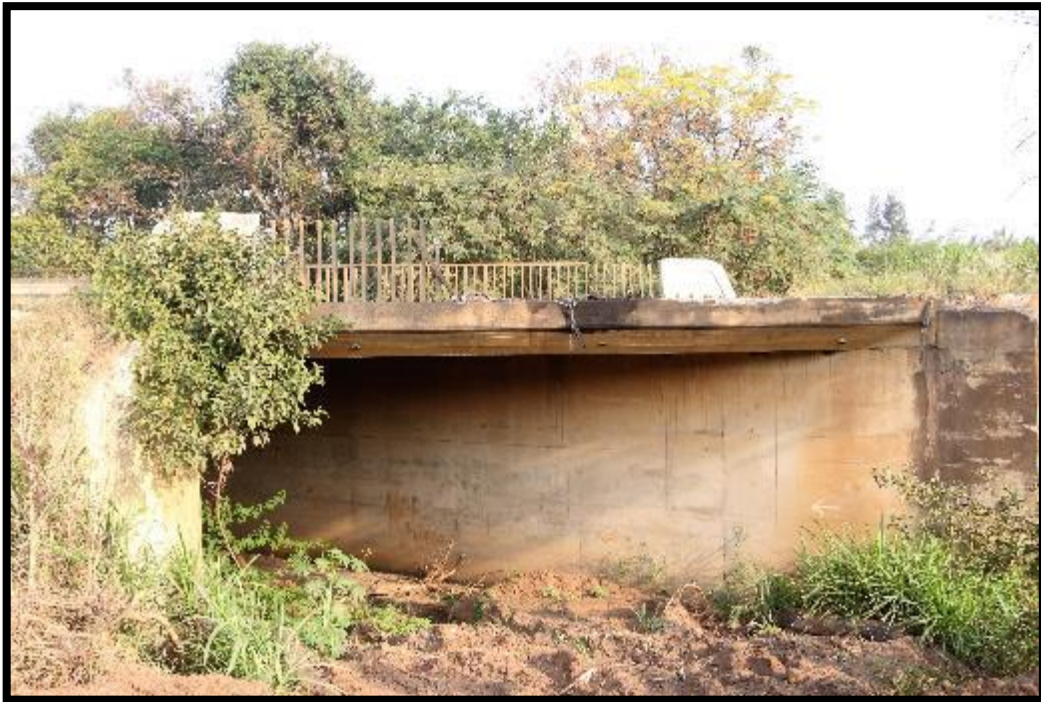
Figure 5: The Bedlane Bridge. Some damage to the existing metal railing is visible.
