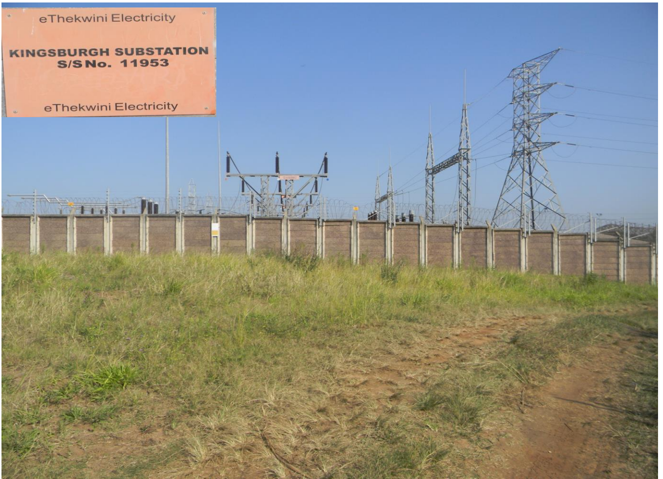
Plate 2: Photo 2: View of Kingsburgh Substation where the proposed powerline will connect (Photograph © by Author 2019).
